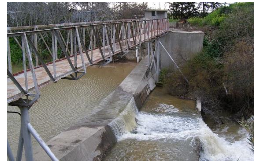
Flow gauging station on Ezousa River near Akhelia. Photo: Gerald Dörflinger; date: February 2009
